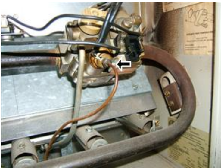
14.7 GAS PIPING Picture 1
